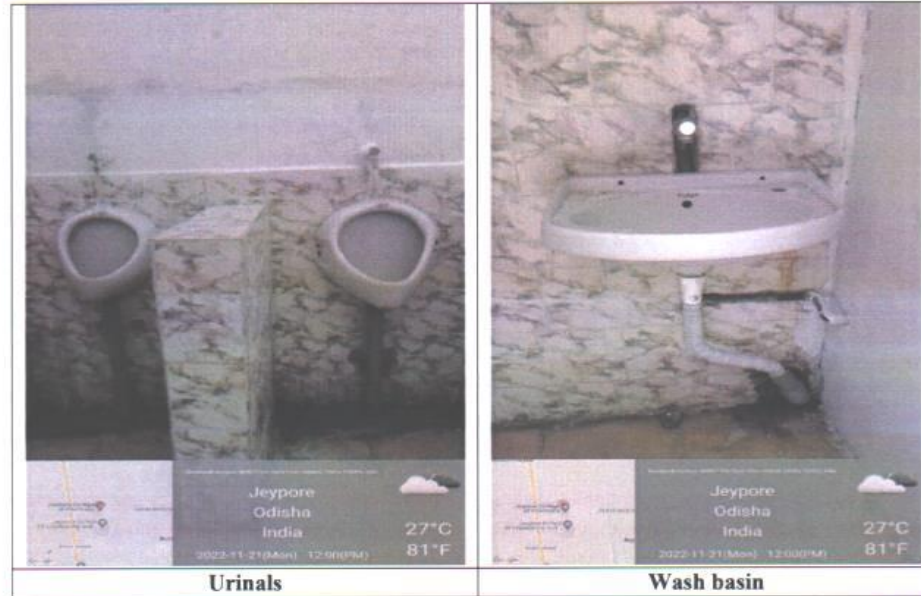
Fig:- 2.6 Urinal & washbasin in college campus
