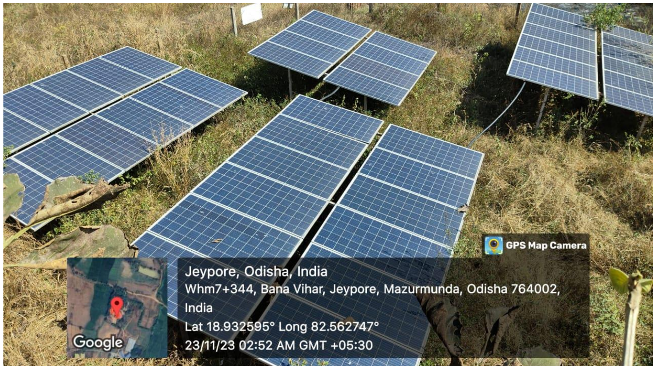
FIG-1 15 KW SOLAR PLANT
